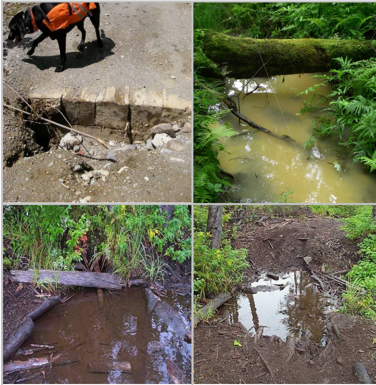
Figure 4: A) Erosion around bridge structure resulting in large inputs of sediment to stream; B) Decreased water clarity downstream of a crossing; C) Accumulation of sediment on the stream bottom downstream of a crossing; D) Disturbance of a stream bank (lack of vegetation, ruts, and tire tracks)
